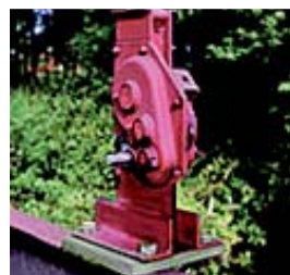
Single Sluice Gate drive
